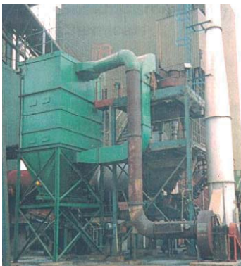
Conveying and Transferring chrome ore at high temperatures
