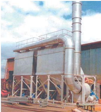
Fume extraction from hot-dip galvanizing process
