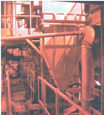
Cement outloading and conveying for production and distribution
